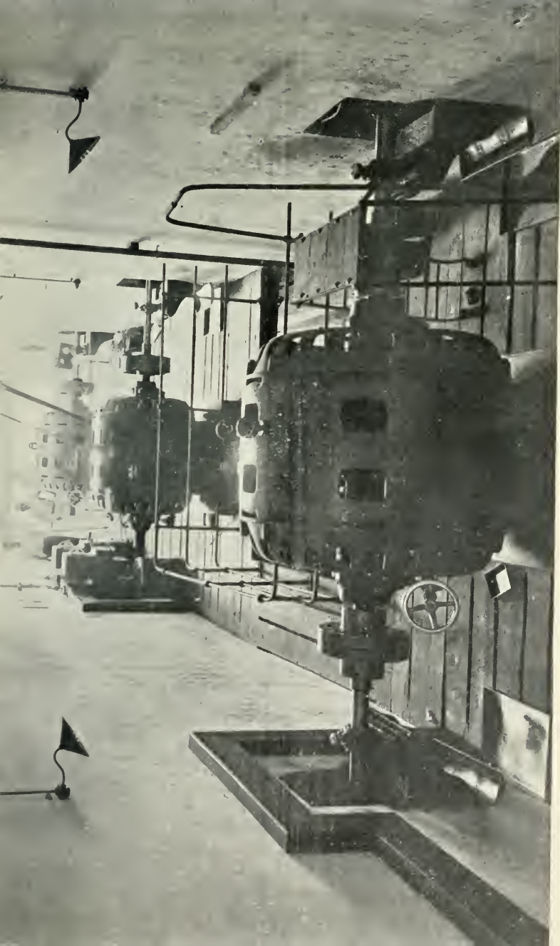
Electric Motors coupled to and driving the shafting in the Simplex Mill.
